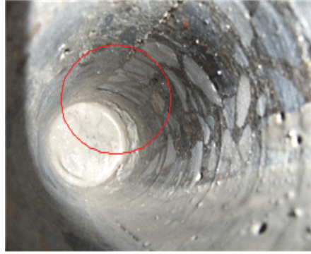
Fig. 4. Void in the interface of sleeper and TCL
